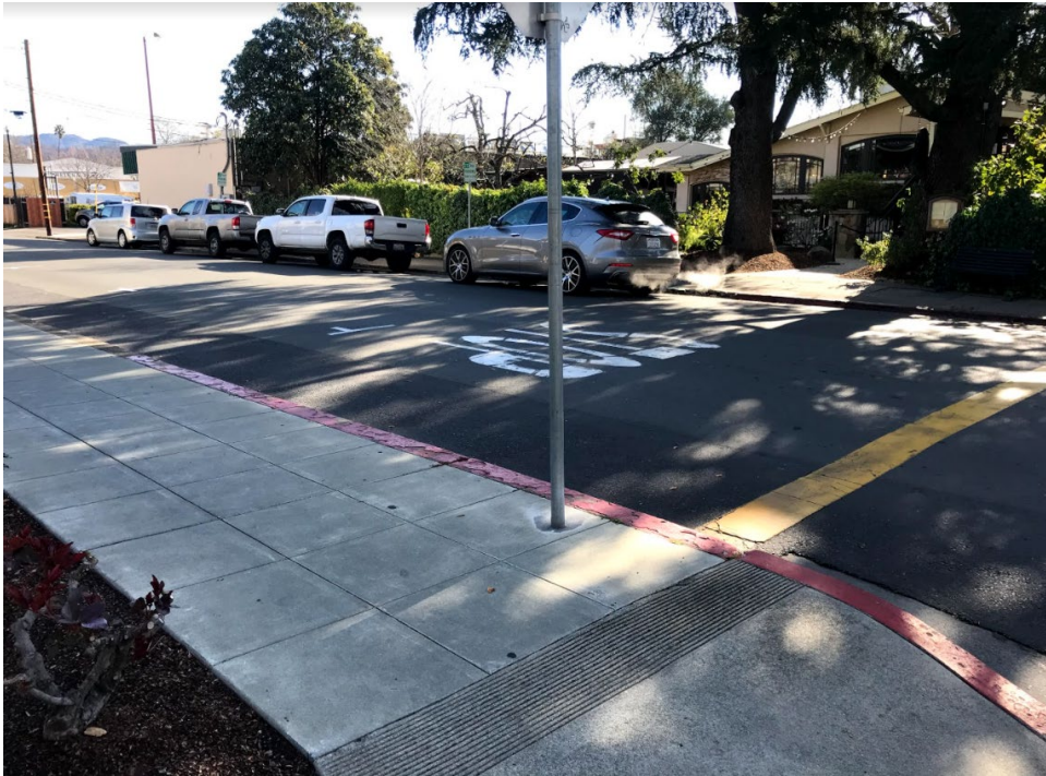
Spring St and Oak Ave: Advanced warning pavement “STOP” marking is too close to the intersection. The narrow road is configured with street parking along both sides, creating visibility challenges for pedestrians in crosswalk.
