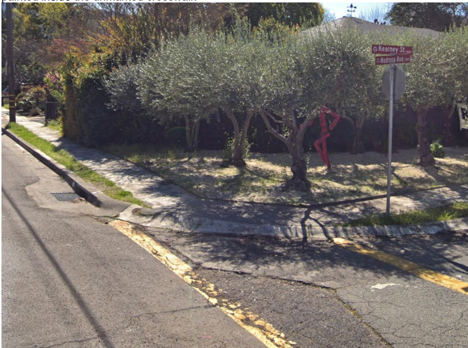
Kearney St and Madrona Ave: Sidewalks are substandard widths, cracked and challenging pavement conditions are present in the crosswalk, and the curb ramp is not ADA compliant.
