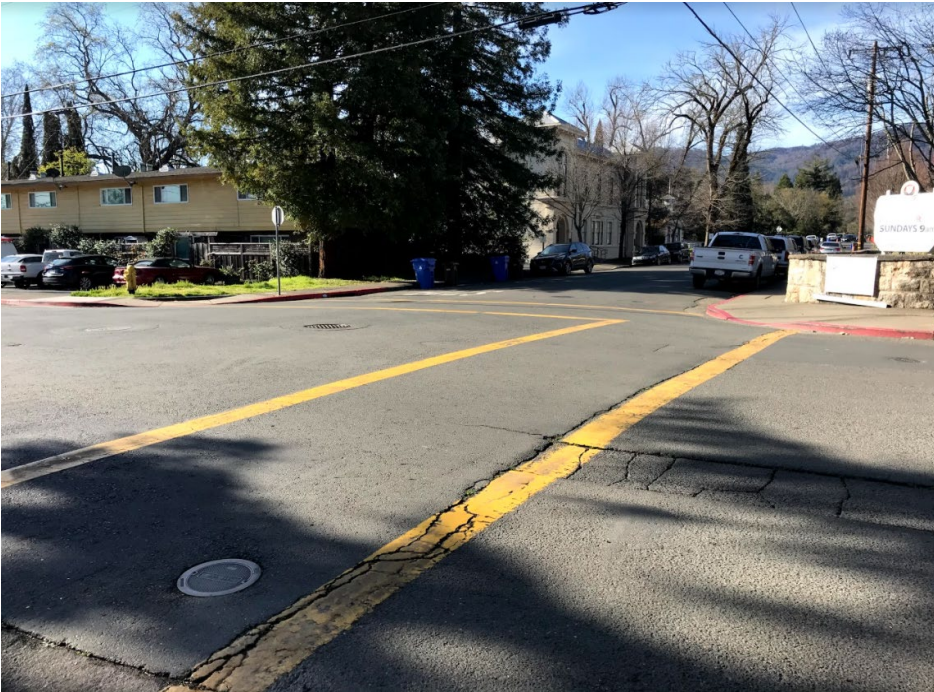
Spring St and Oak Ave: Challenging pavement conditions in crosswalk for ADA users, curb ramps are not ADA compliant due to abrupt level changes between the gutter and ramp.
