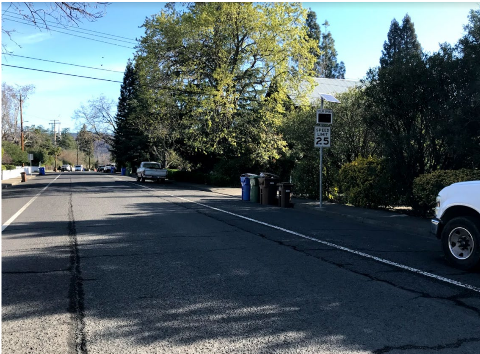
Spring St: cracked and deteriorating pavement presents challenges to bicyclists. Some efforts have been made to reduced speeding along this roadway (see radar speed feedback sign), but more traffic calming is needed.
