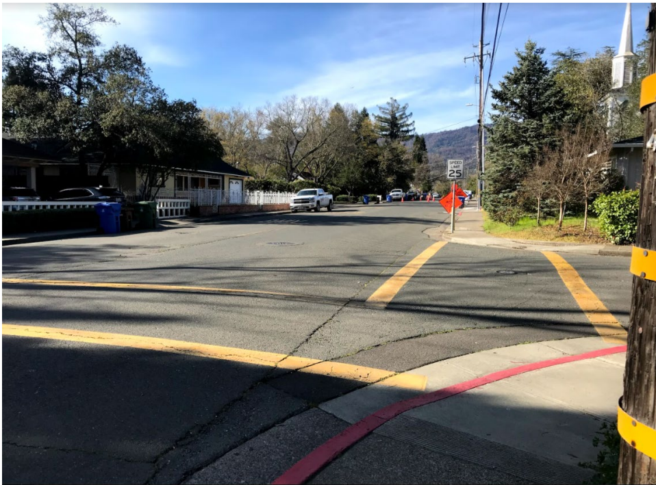
Spring St at Kearney Ave: Pavement conditions in the crosswalk present challenges to pedestrian and ADA users, with challenging slopes, cracked pavement, and curb ramps that are not ADA compliant.
