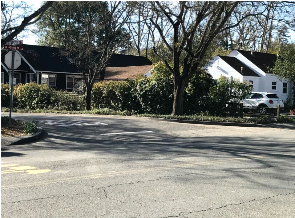
Spring St and St. James Dr: Example of unmarked crosswalks near the School Zone, Stop Bar is too close to the intersection, and pavement conditions in crossing present challenges
