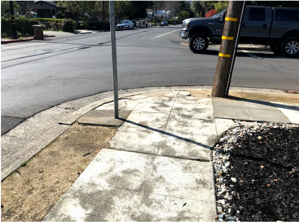
Spring Mountain Rd and Madrona Ave: Example of crumbling, uneven sidewalks and unmarked crossing that lacks curb ramps.
