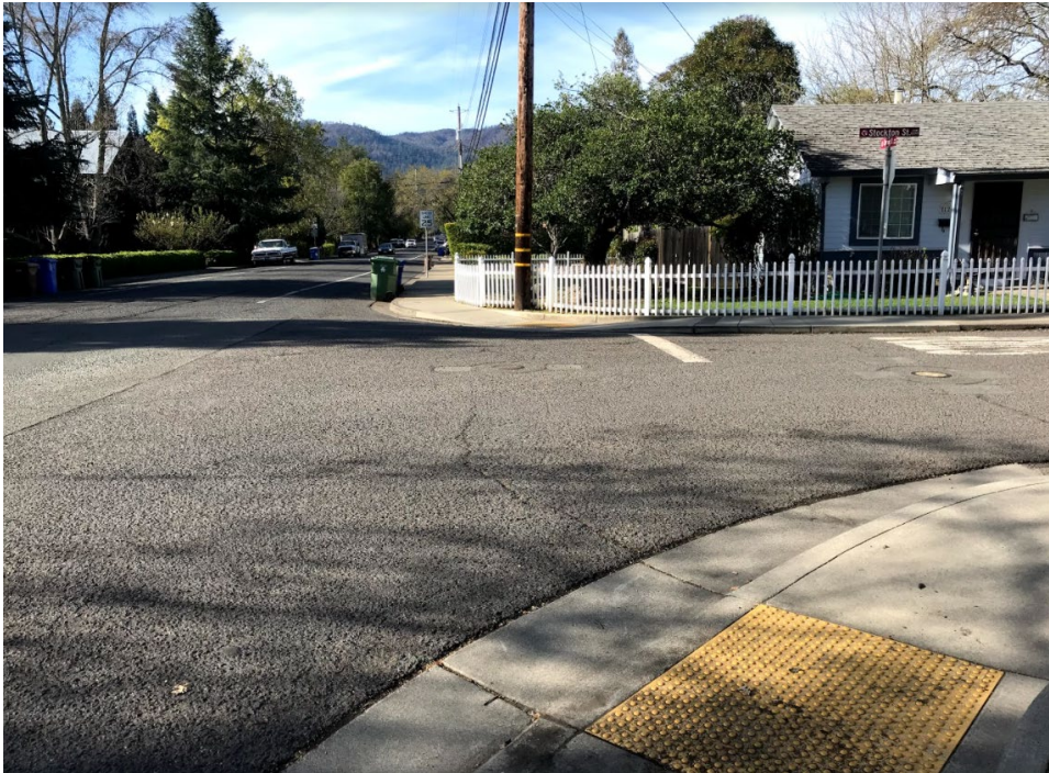
Stockton St and Spring St: Example of unmarked crosswalk, with stop bar too close to crossing zone.
