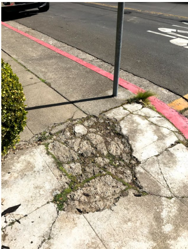
Oak Ave and Madrona Ave: Example of crumbling sidewalk pavement
