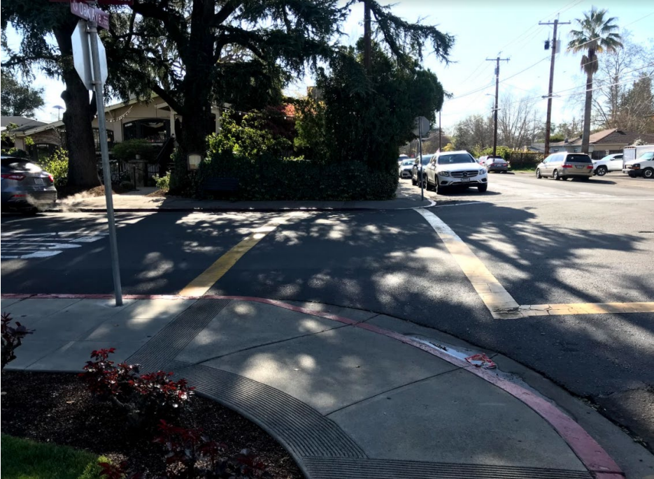
Spring St and Oak Ave: Curb ramps are not ADA compliant, with challenging pavement slope, slope of ramp, and transition between the street and ramps are not flush.
