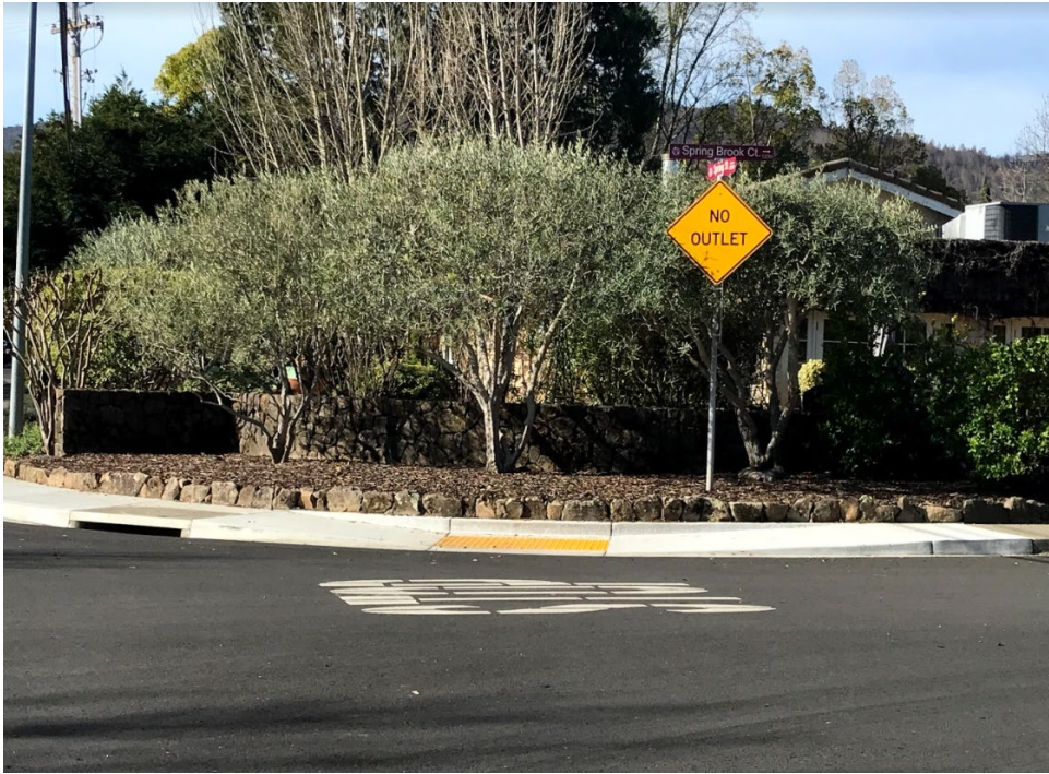
Spring St and Spring Brook Ct: "STOP" Marking is not located in advance of the intersection, it is painted inside the unmarked crosswalk
