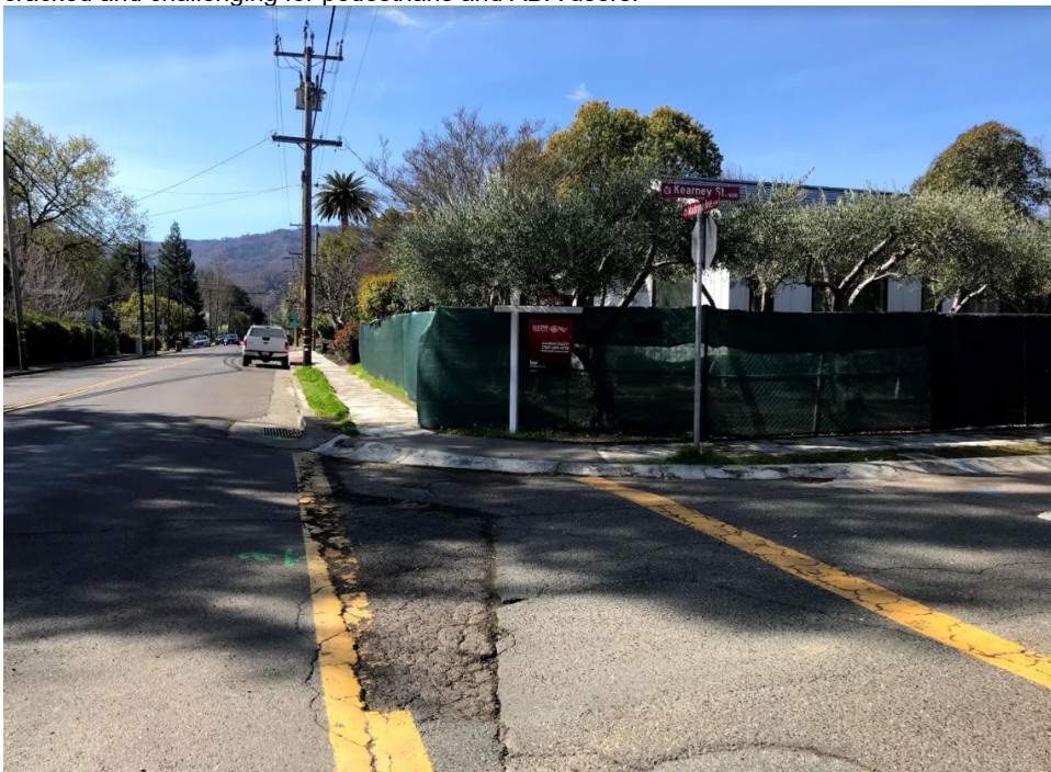
Madrona Ave and Kearney St: Sidewalks are missing curb ramps, pavement in crossings are also cracked and challenging for pedestrians and ADA users. Crosswalk markings need to be repainted.
