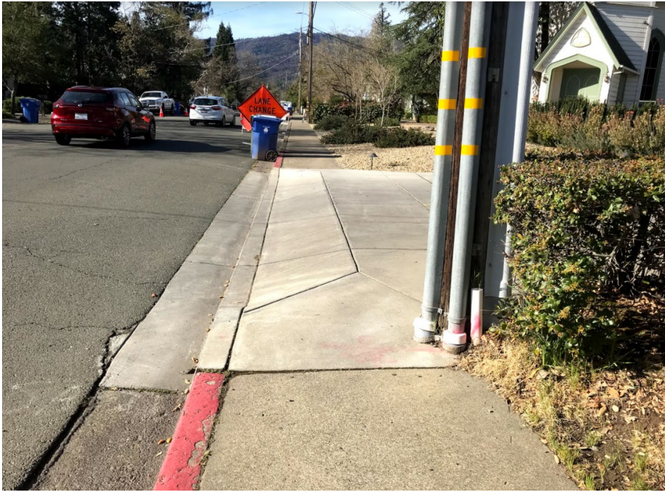
Spring St: Challenging sidewalks for pedestrians and ADA users due to the presence of a steep driveway, the sharp angle to go around it, and the narrow width of the sidewalks.
