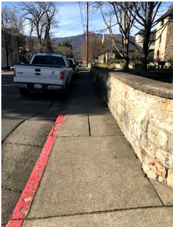
Spring St: Sidewalks are substandard width, with cracked and challenging pavement conditions for ADA users.
