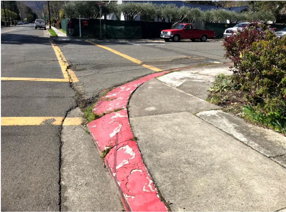
Madrona Ave and Kearney St: Sidewalks are missing curb ramps, pavement in crossings are also cracked and challenging for pedestrians and ADA users.
