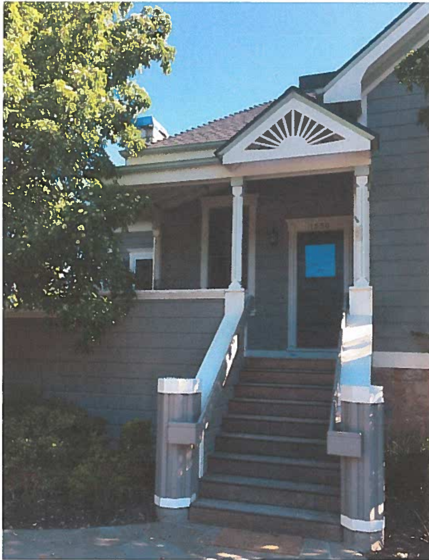
Photo 4: Additional detail of front stairs to be removed/replaced.
