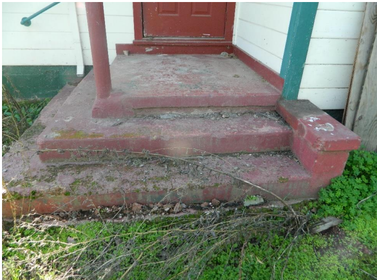
Figure 10. Red-dyed front porch stoop and stairs.
