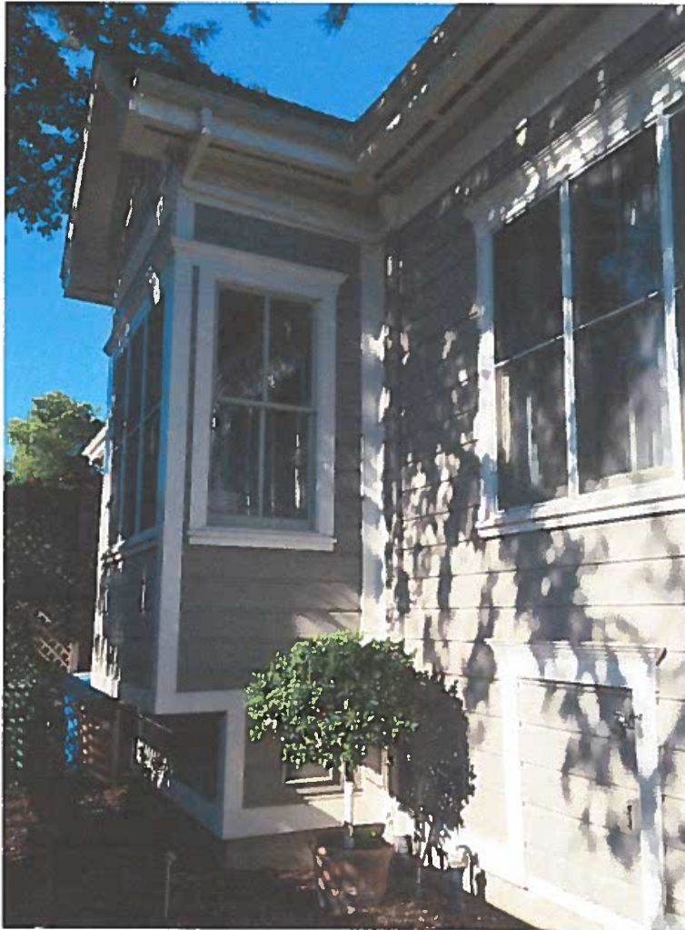
Photo 2: Side/South Elevation – location of proposed 100 sf deck.
