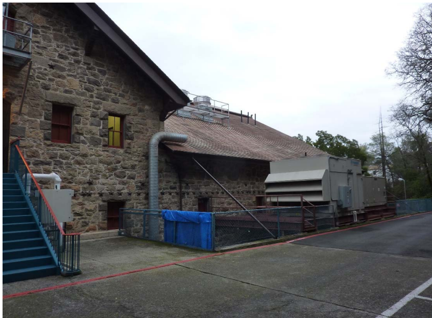
Image 6. Existing mechanical equipment – View from northwest
