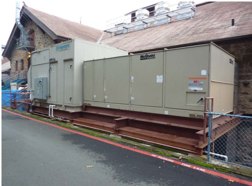
Image 5. Existing mechanical equipment – View from southwest
