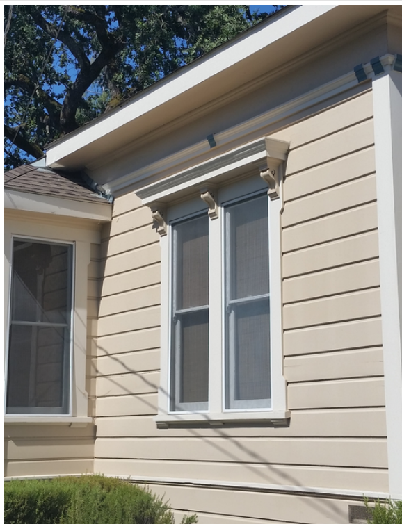
Figure 4. Typical “hooded” window (pair) on twin house next door. Note the “chopped” corbel remnants above.
