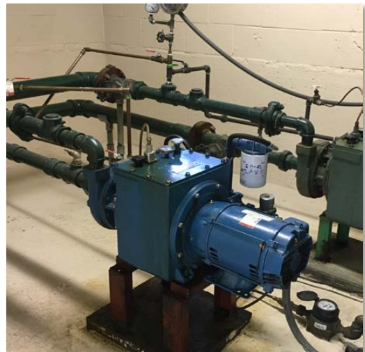
Figure 1.1 Pump Station at the Water Treatment Plant. Estimated project cost of $200,000
