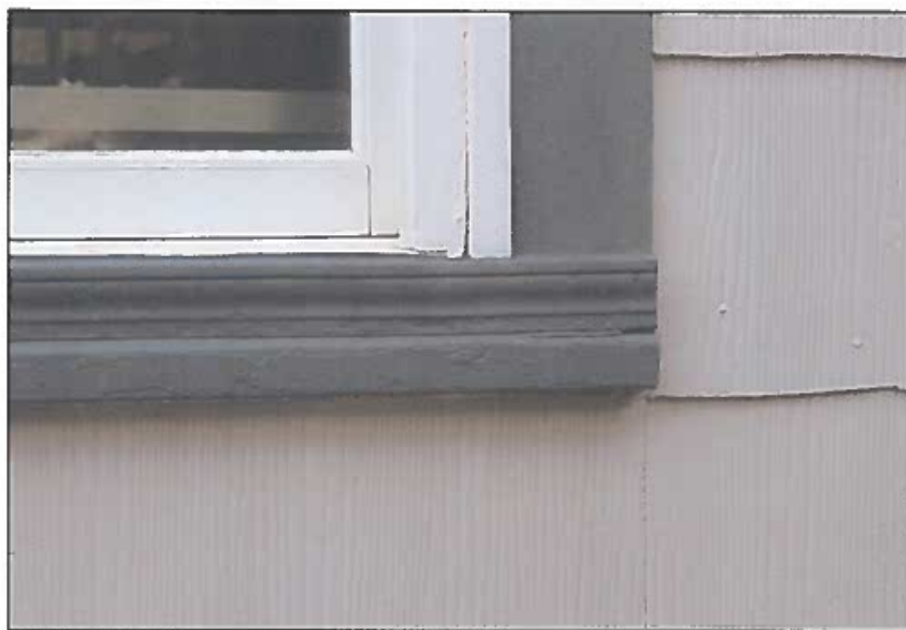
Figure 19: Modified trim on replacement window on rear gable
