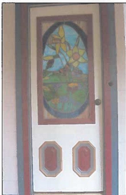
Figure 8: East elevation, modified original door inside screened porch
