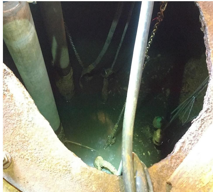
Wet Well Access Hole
