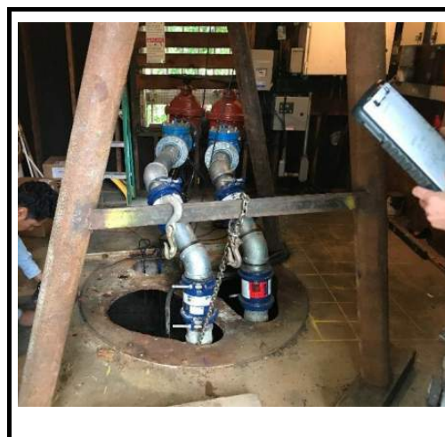
Right Hand View of Pump
