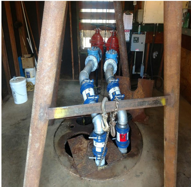
Wet Well Discharge Piping
