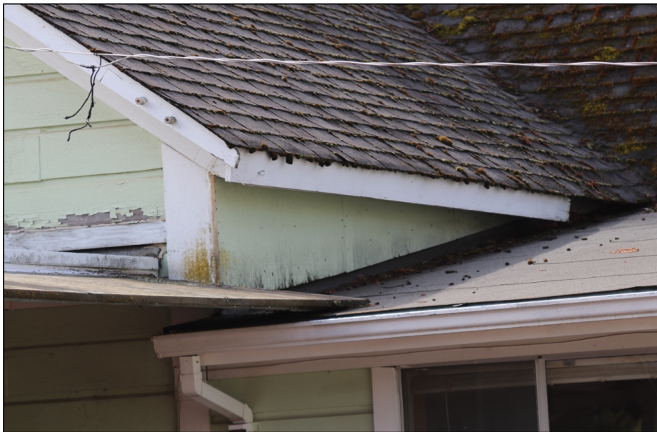
Figure 14: North elevation, plywood patch at roof junction
