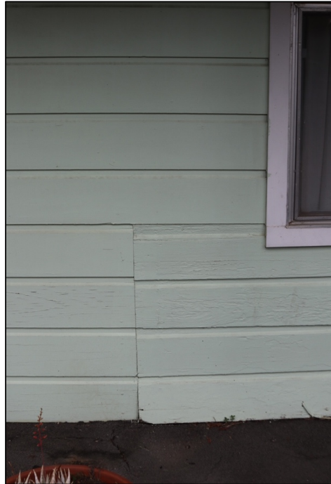
Figure 5: South elevation, infilled porch, patched siding
