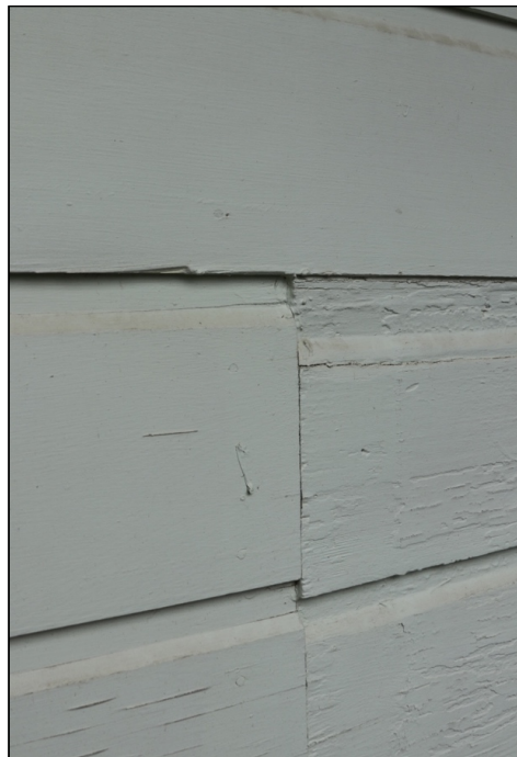
Figure 6: South elevation, detail of patched siding
