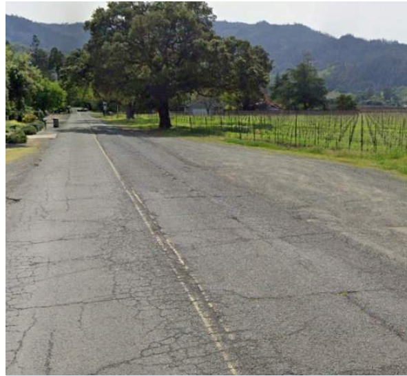
Sulphur Springs Avenue Roadway Condition (2024)
