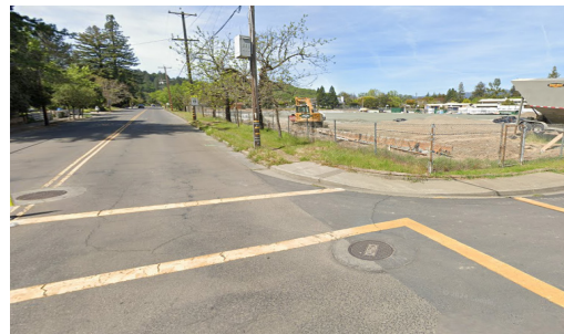
Most curb ramps are not currently ADA-compliant
