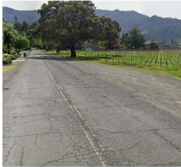
Sulphur Springs Avenue Roadway Condition (2024)
