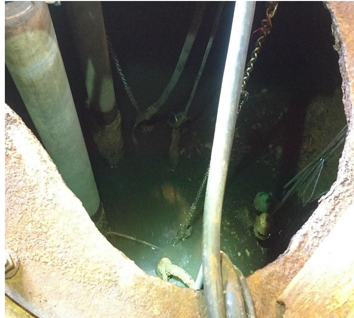
Wet Well Access Hole
