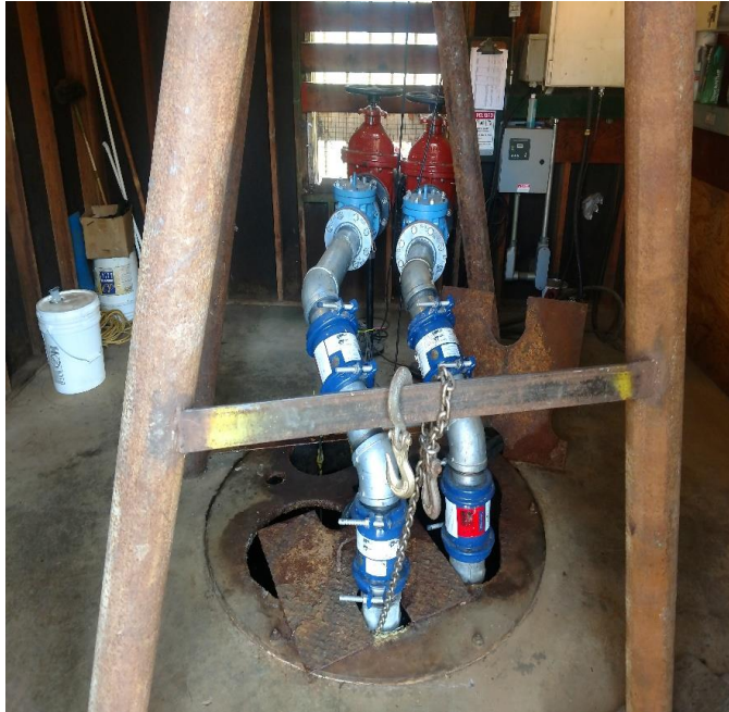
Wet Well Discharge Piping
