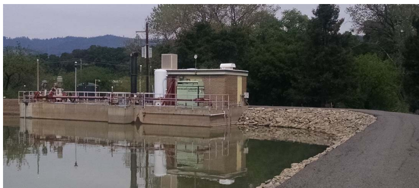
Figure 27 – Chlorine Contact Tank and Effluent Pump Station at Pond 5
