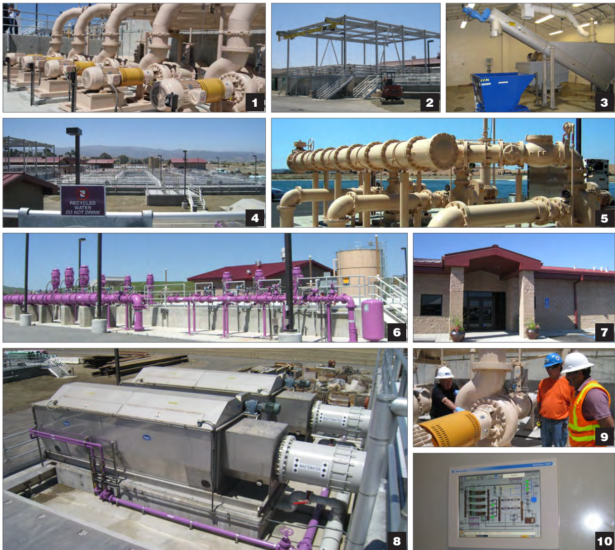
1 Mixed liquor pumping station 2 Membrane filtration with bridge crane system 3 Washer compactors 4 Overview of MBR aeration basins 5 Influent pump station 6 Plant water pump station 7 Operations and maintenance building 8 Influent screens 9 Construction management and operations staff inspecting a pump 10 Local control panel operator interface
