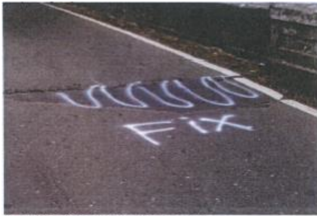
A section of the roadway has settled.
