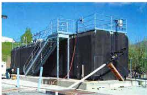
ISAM™ Packaged Sequencing Batch Reactor
