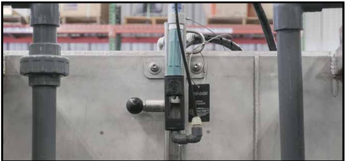
Example Sensor Installation
