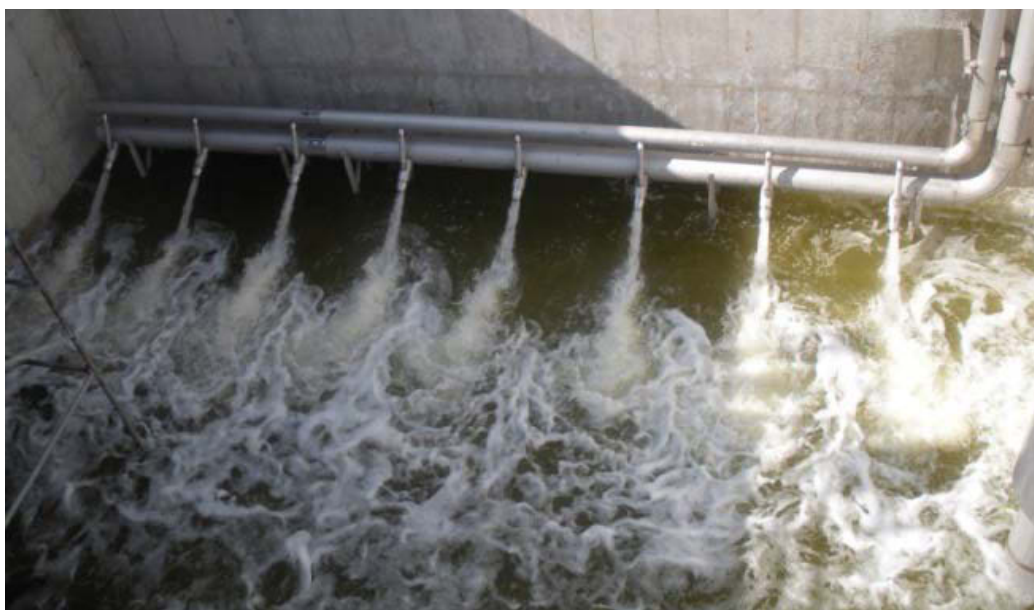
Stainless steel jet aeration header
