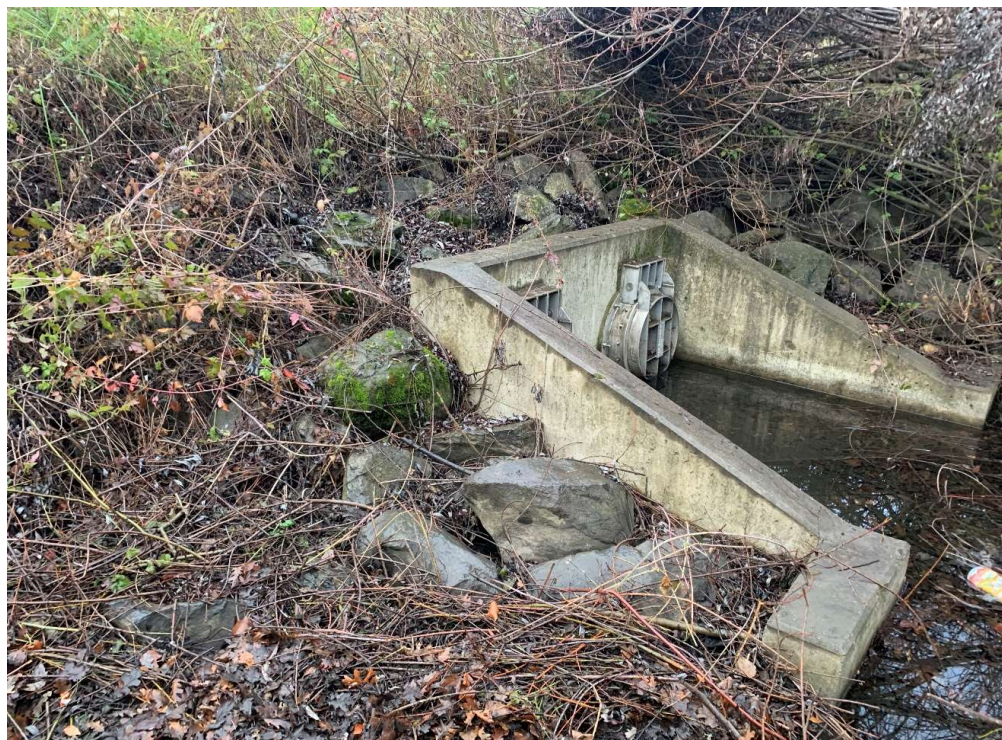
Pump Station Photo 7: Pump station discharge pipes concrete outfall structure with flap gates.
