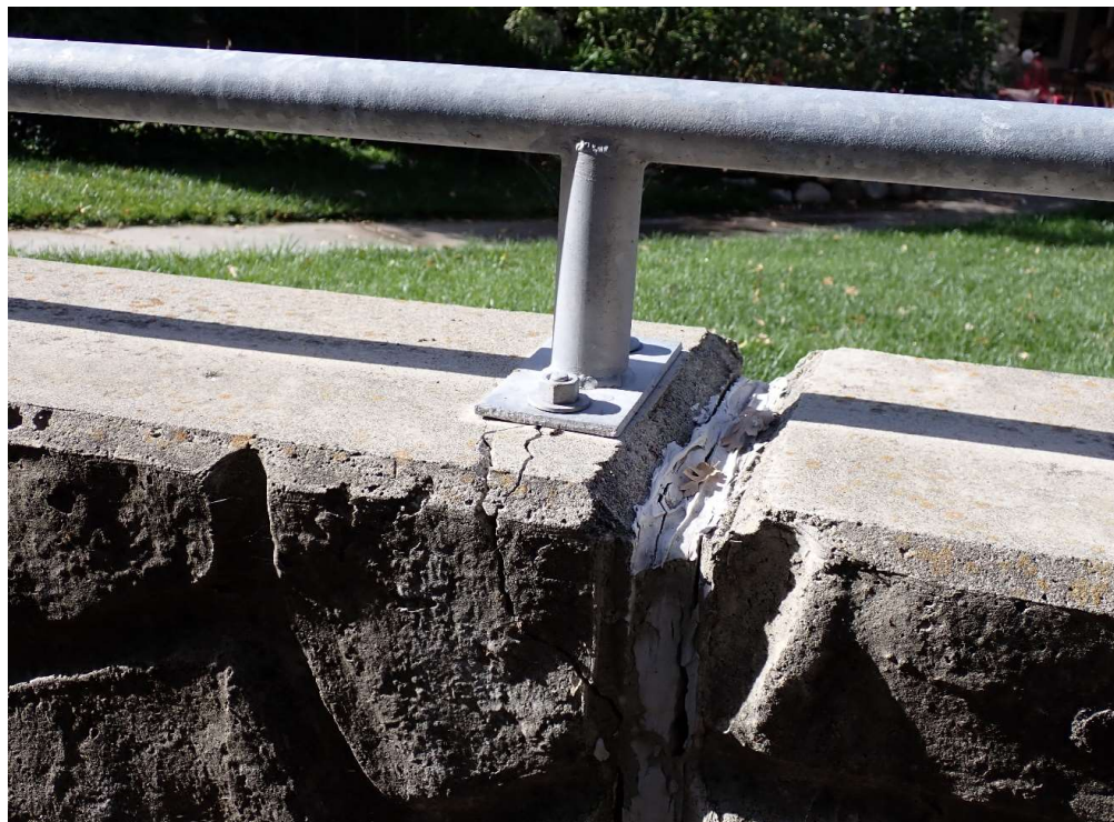
Floodwall Photo 3: Floodwall crack at handrail baseplate (waterside pictured)
