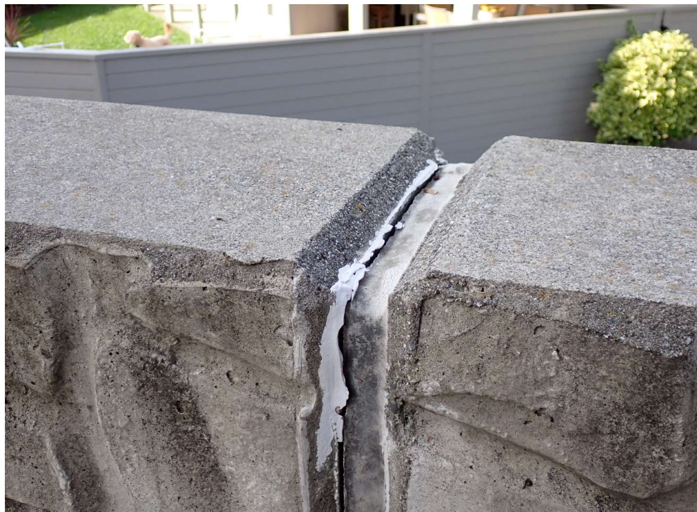
Floodwall Photo 2: Typical floodwall joint with caulking separation and previous repair work.
