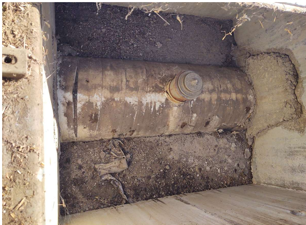
Pump Station Photo 6: West pump station discharge pipe inside valve vault with pipe tape wrap peeling off.
