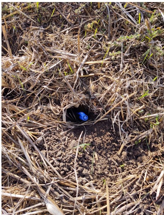
Levee Photo 3: Typical rodent hole less than 3" in diameter and less than 6" deep.
