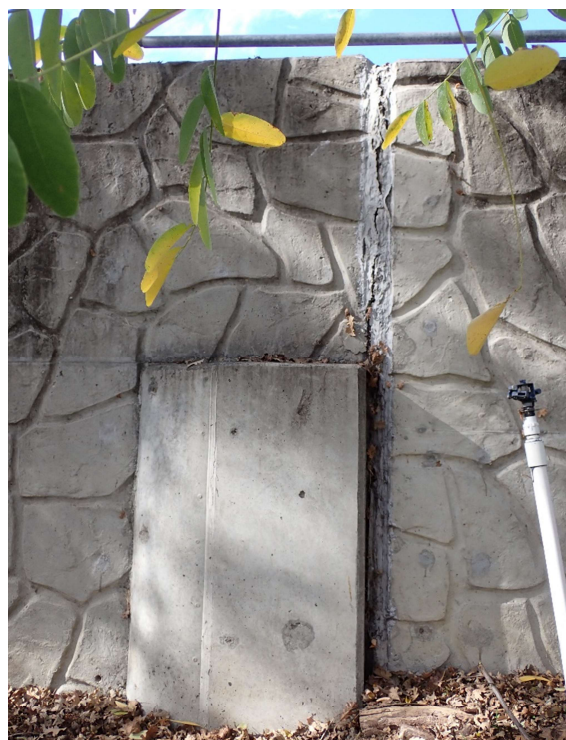
Floodwall Photo 8: Joint movement at interface of T-wall and I-wall, Sta 37+23.5 (waterside pictured)
