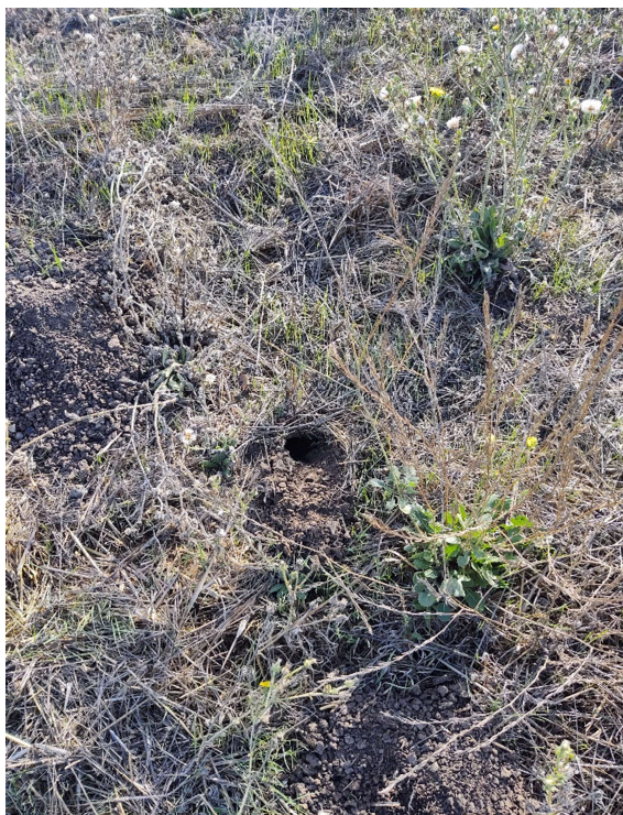
Levee Photo 5: Typical rodent hole less than 3" in diameter and less than 6" deep.
