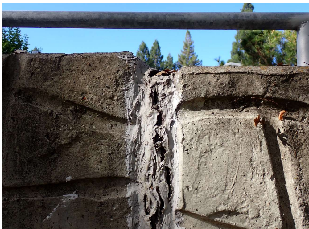
Floodwall photo 9: Joint movement at interface of T-wall and I-wall, Sta 37+23.5 (waterside pictured)
