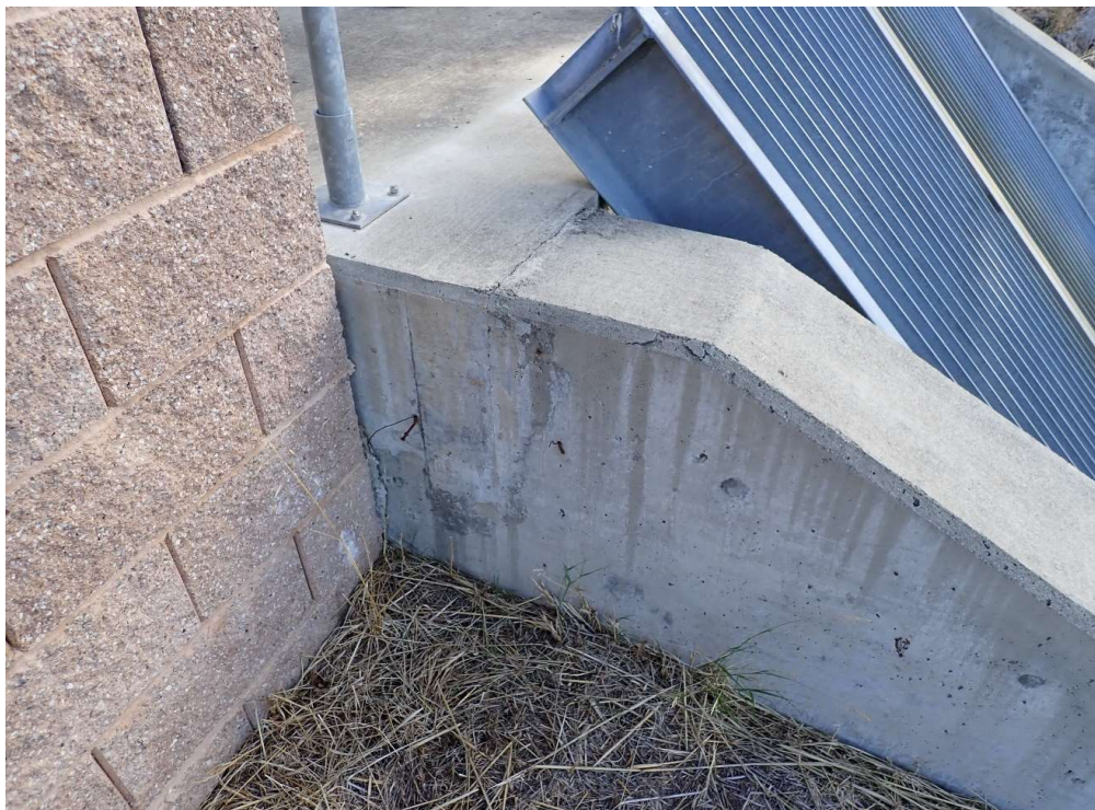
Pump Station Photo 3: Minor cracking along interface of pump sump elevated deck and wingwall with visible concrete repair work.
