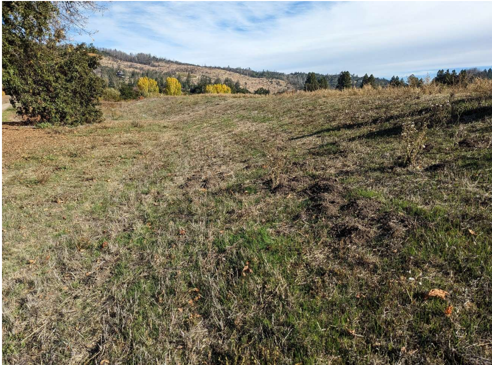
Levee Photo 7: Rodent activity on waterside of levee near the Oak trees adjacent to the storm drain outfall to terrace excavation.
