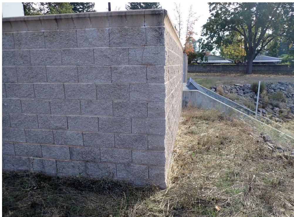
Pump Station Photo 5: Southwest corner of CMU perimeter wall cracking.
