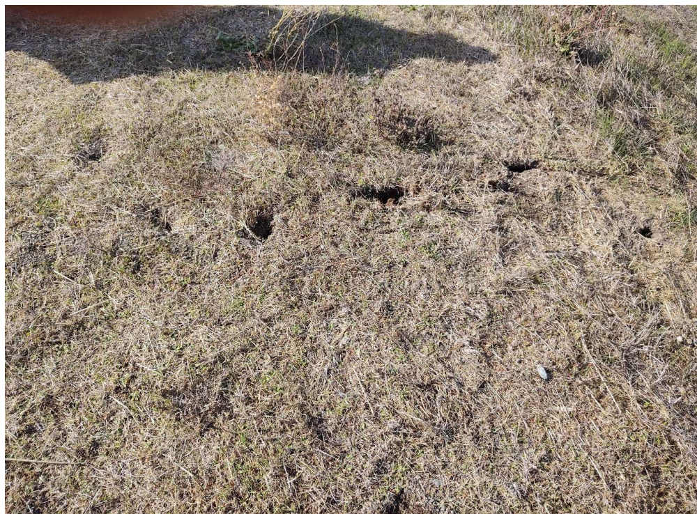
Levee Photo 4: Typical rodent holes in top of levee. Holes are less than 3" in diameter and less than 6" deep.
