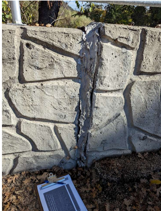
Floodwall Photo 5: Joint movement at interface of T-wall and I-wall, Sta 37+23.5 (landside pictured).
