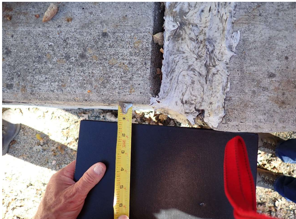
Floodwall Photo 7: Joint movement at interface of T-wall and I-wall, Sta 37+23.5. Measured approximately 1.25" horizontal offset.
