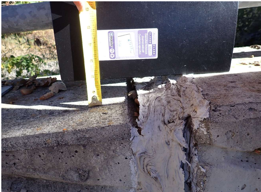
Floodwall Photo 6: Joint movement at interface of T-wall and I-wall, Sta 37+23.5. Measured approximately 1.5" vertical deflection.
