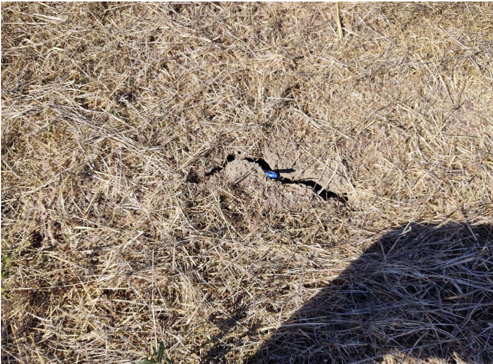
Levee Photo 8: Typical minor dessication crack on the landside of the levee, less than 6 inches in depth.
