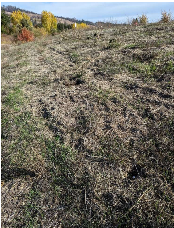
Levee Photo 6: Typical rodent hole less than 3" in diameter and less than 6" deep.
