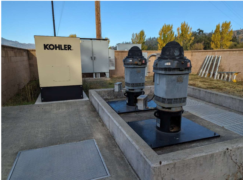
Pump Station Photo 1: Lead and Lag Pumps, with Kohler generator and control panel in the background.
