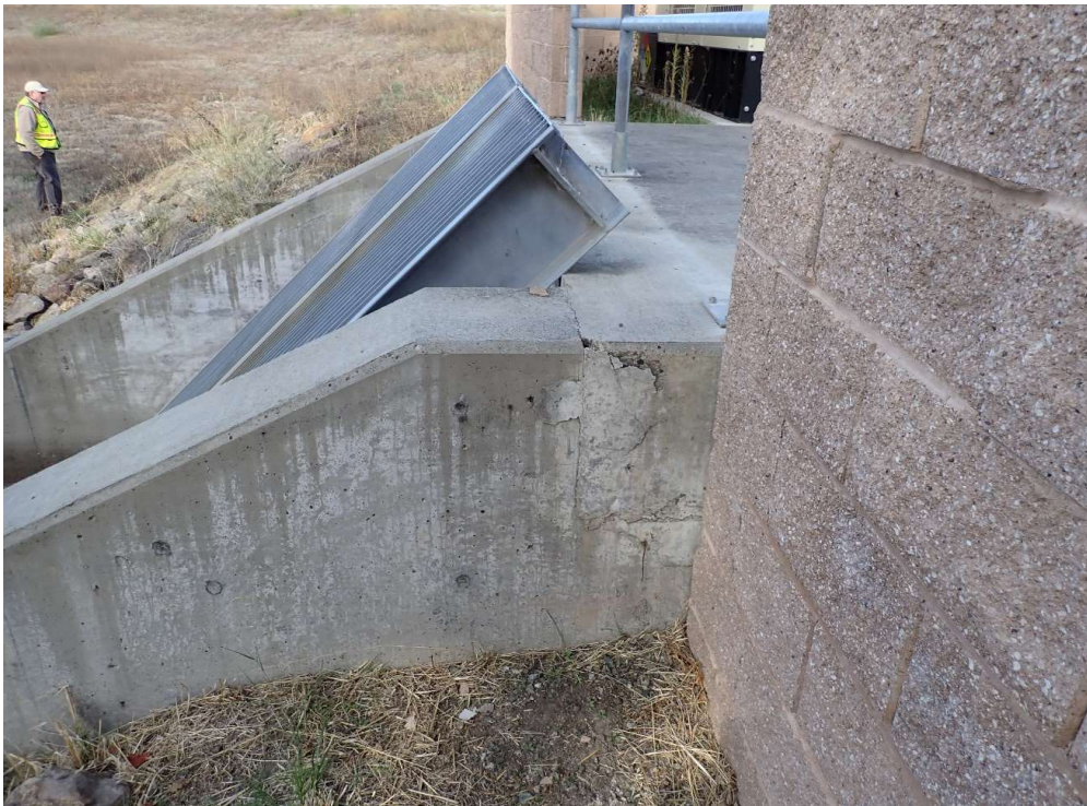
Pump Station Photo 2: Minor cracking along interface of pump sump elevated deck and wingwall with visible concrete repair work.
