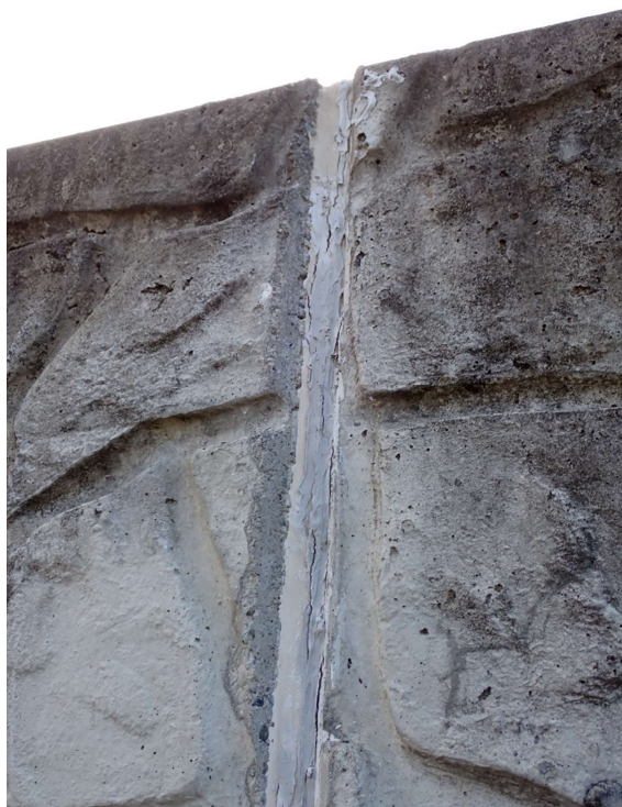
Floodwall Photo 1: Typical floodwall joint with caulking separation and previous repair work.
