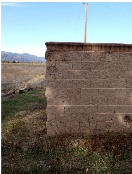
Pump Station Photo 4: Southeast corner of CMU perimeter wall cracking.
