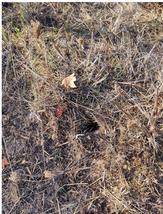
Levee Photo 2: Typical rodent hole less than 3" in diameter and less than 6" deep.
