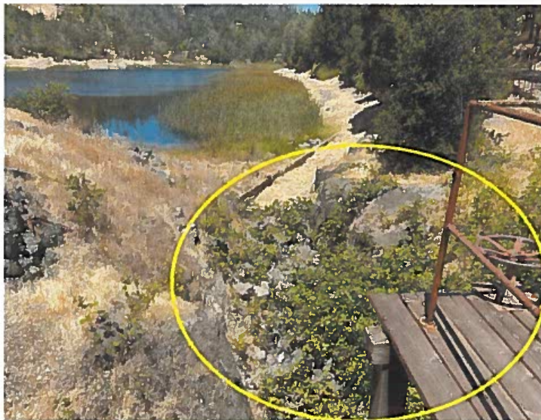
Photo 4: View of spillway approach and control looking upstream. Remove berry vines (circled).
