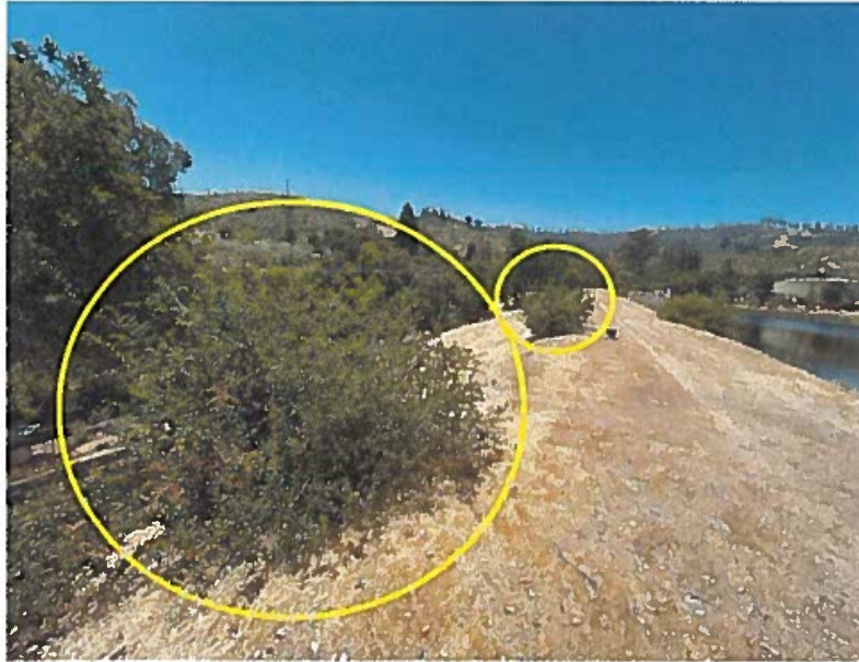
Photo 7: Remove woody vegetation from the downstream slope (circled).
