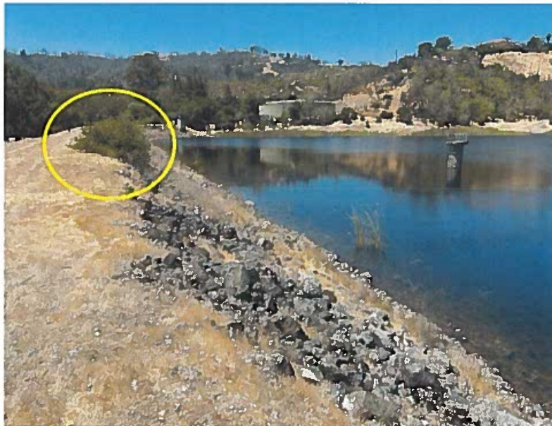
Photo 6: Remove woody vegetation and minor tule growth from the upstream slope (circled).
