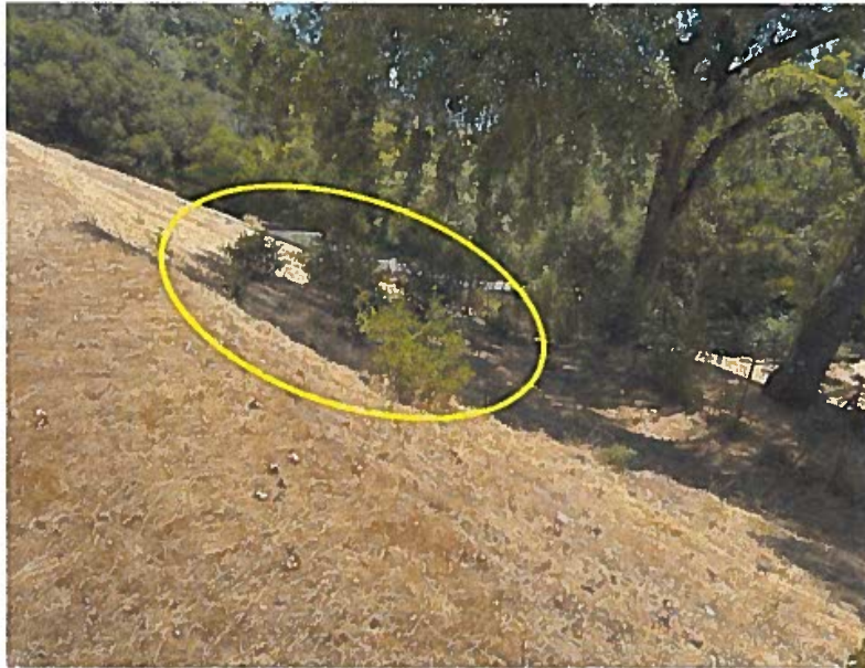
Photo 5: Remove vegetation from the downstream slope (circled).
